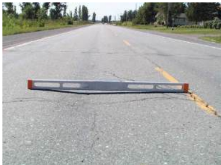
(a) Rutting damage.
