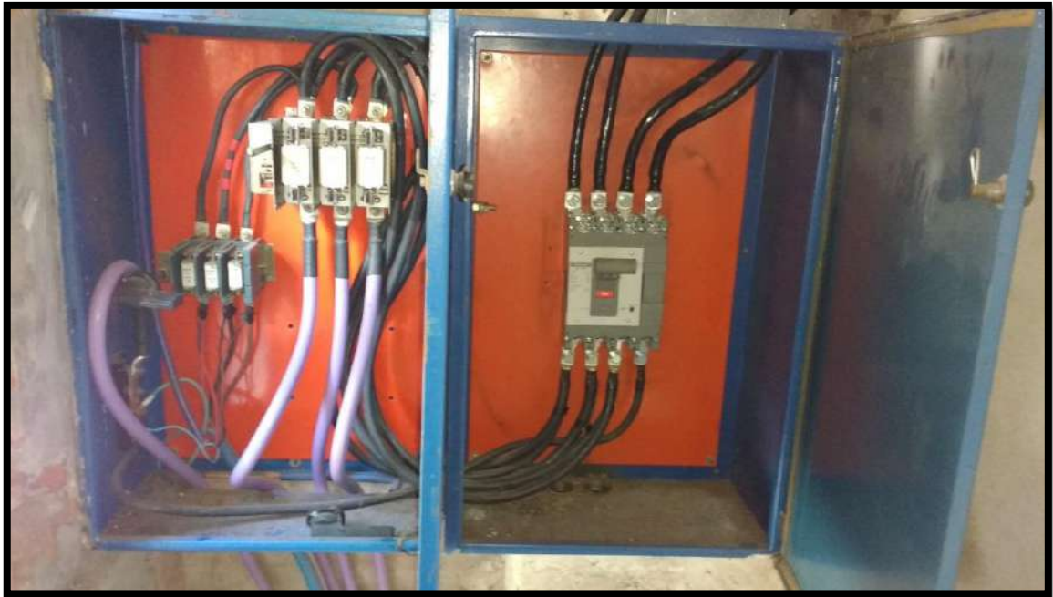
Fig. 7.13. Interior de tablero TG5-0
